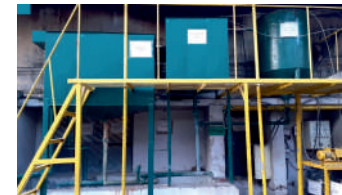
ETP Water Treatment plant
