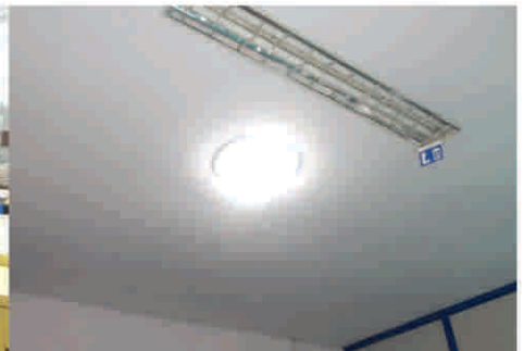
Day Light Harvesting system at our work place
